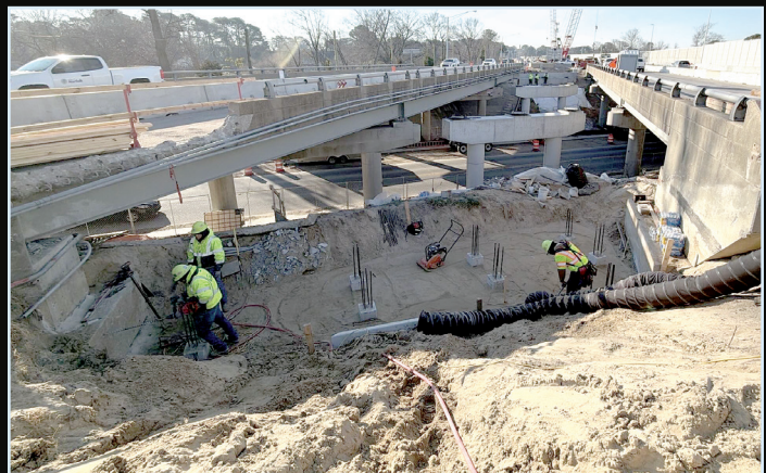
Working between two existing bridges, crews work to place the foundation to widen the westbound bridge over 1st View Street.
