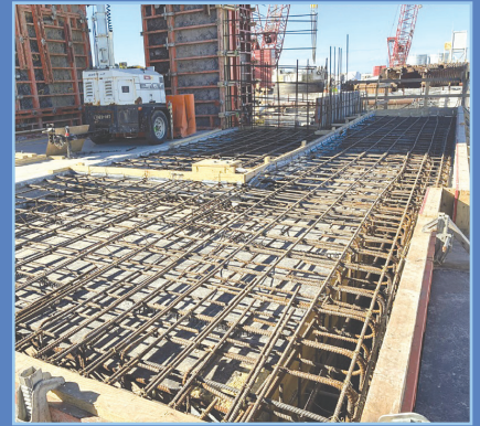
The buildings are supported by a foundation of reinforcing steel and concrete.
